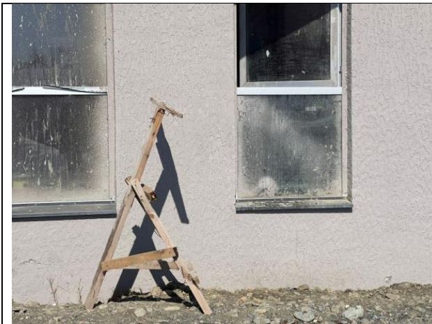
Not supported slab (2) self made platform in hazardous zone (3) Self made hanging platform - critical inconsistency
