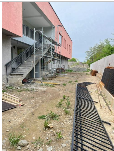
Status: (open, In progress, closed) - Open
