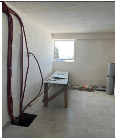
Status: (open, In progress, closed) - Open
