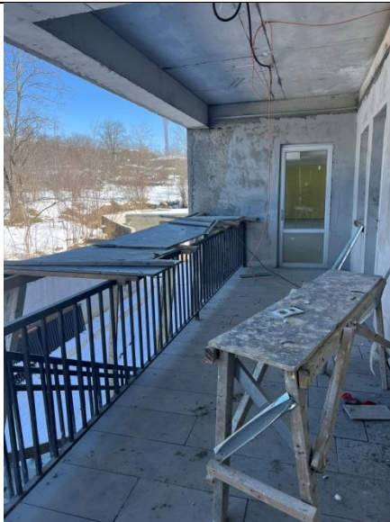
Self made "scaffolds" detected
