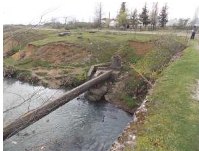
Picture 4.1.2 Untreated Wastewater Discharge Point
