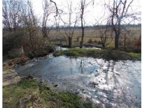
Wastewater flowing out from damaged pipe
