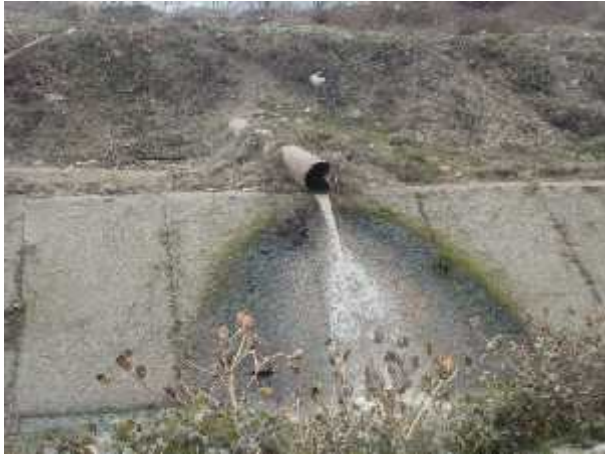
Wastewater discharge point into irrigation channel
