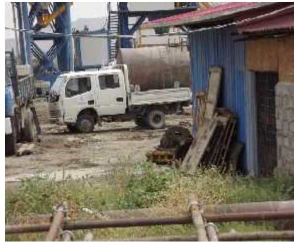
Construction camp Containers with hazardous materials have been removed to covered building
