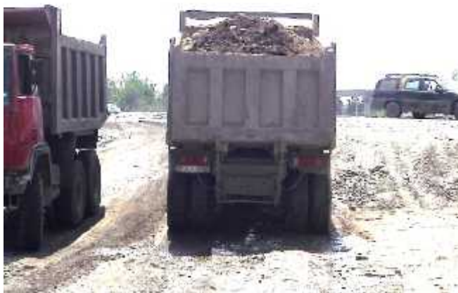
Contractors trucks, transported loose materials are not covered
