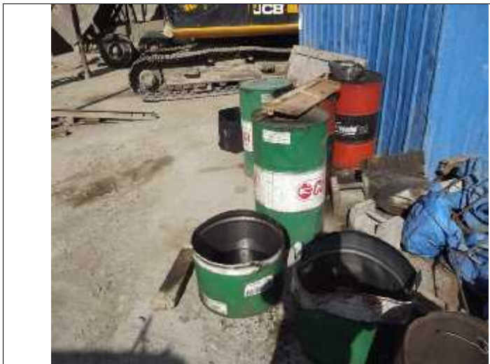
Construction camp Disposal of oil products without drip trays
