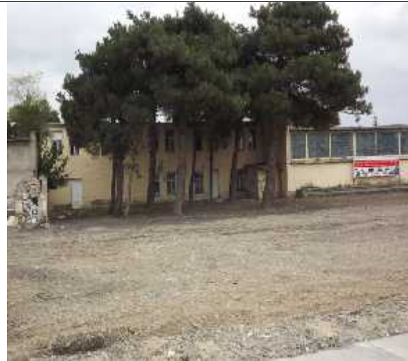
PK120 Milled asphalt was removed and used for paving of access roads
